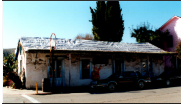
Maintenance on historic structures can be costly
